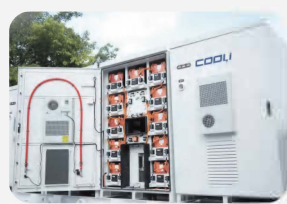
Energy storage container
